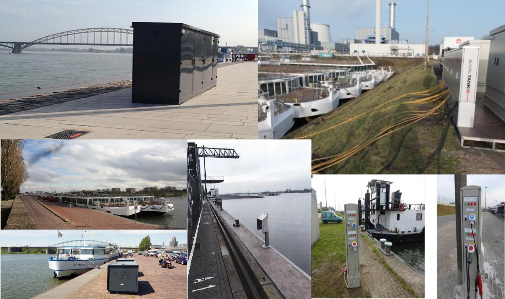
Overview of different types of OPS equipment in NWE region
